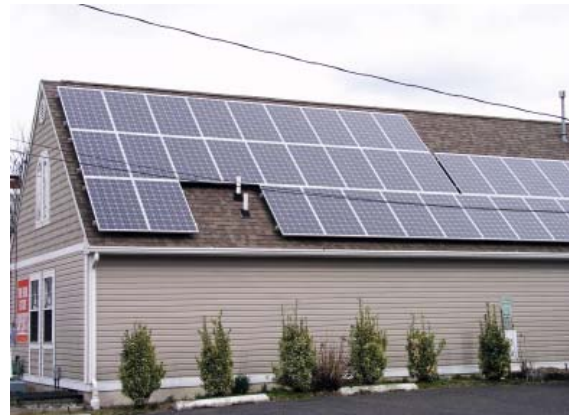
Recent changes to Pinelands rules provide a mechanism to speed the development of accessory solar energy facilities such as the one above.
